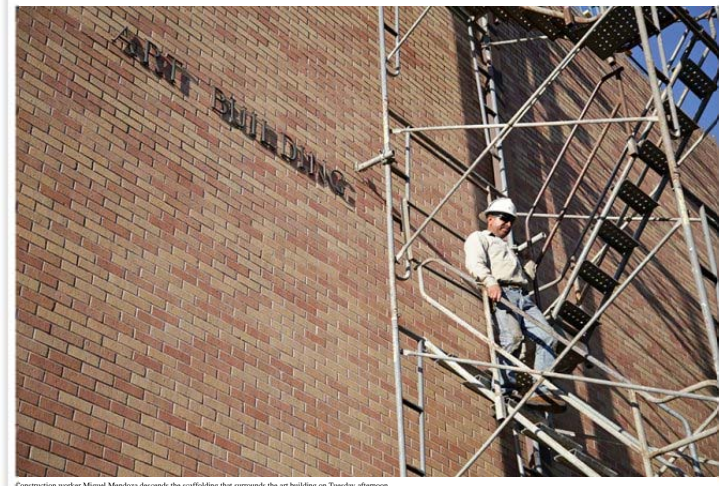
Construction worker Miguel Mendez descends the scaffolding that surrounds the art building on Tuesday afternoon. Photo Credit: Marshall Trickett (author/marshall-trickett) | Daily Texan Staff
